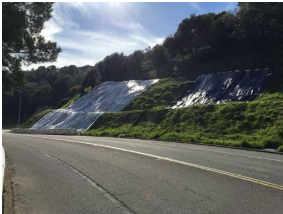
Landslide sites on Andersen Drive with tarps for temporary weather protection
